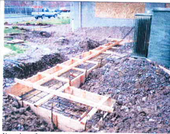
Footing form ready for concrete south of Music Room, masonry wall not started, 3-27-09.
