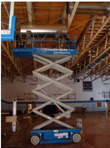
New Ductwork in Main Gym
