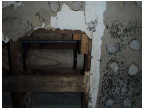
Glue Dots and Old Drain in South Hall
